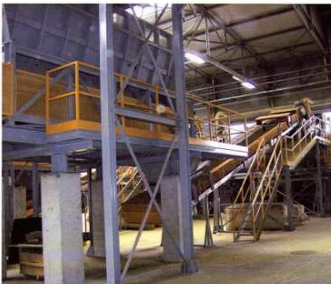
Laminatoi a monte delle due mattoniere. Rolling mill upstream of the two brick-moulding machines.
